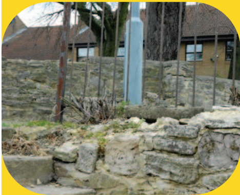
Vandalised wall at the rear of Dorset Place Community Centre.
