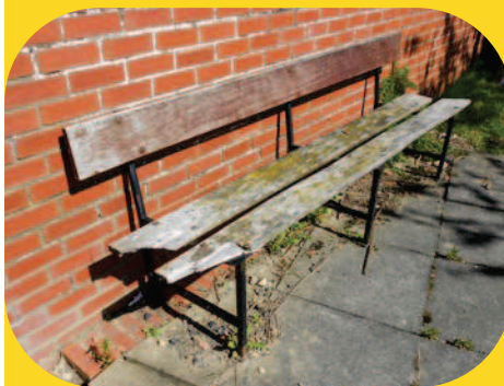
Dilapidated bench in Dorset Place.
